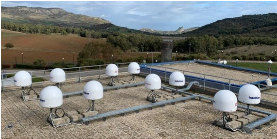
Picture 1: enterprise rooftop-mounted OneWeb user terminals
